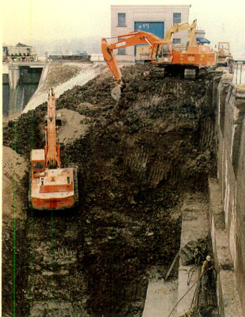
Welland Canal Rehabilitation Program: Workmen prepare site prior to strengthening the east wall of Lock 3. The work was done last winter.
