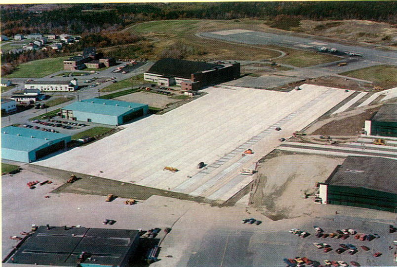
Concrete paving laid by Standard Paving Maritime Limited at Shearwater, Nova Scotia, Armed Forces Base.
