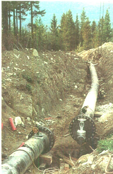
A section of pipe is exposed for inspection and repair at Jackman Hill in the Canadian Rockies.
