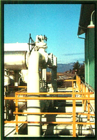
(top) Broadway Plaza in Vancouver houses the offices of Trans Mountain's administrative, engineering, oil movements and management staff.
