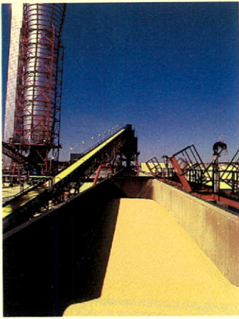
North America's first sulphur prilling tower, at Strachan Gas Plant, makes a low-dust product popular with shippers.
