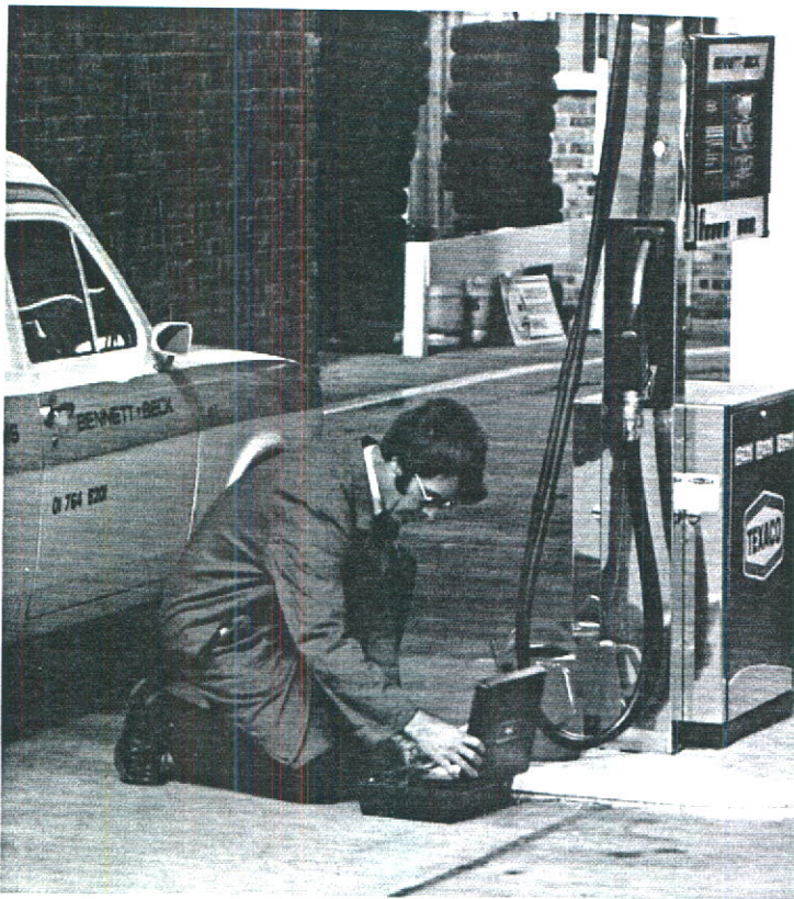
Bennett Pump engineers provide final hook-up and testing services for all new installations.
