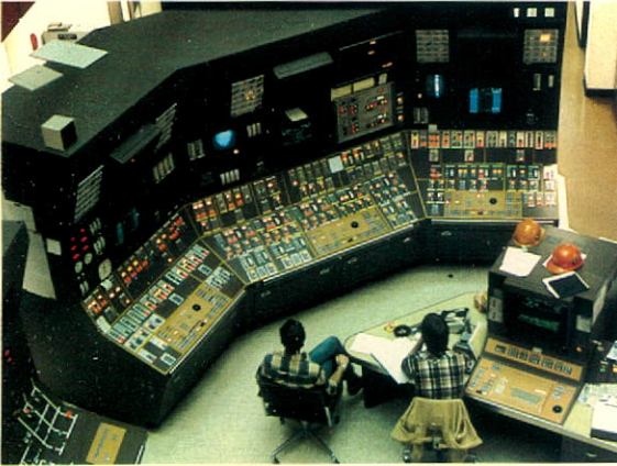
The Thunder Bay Generating Station is the first fully automated generating plant in North America.
