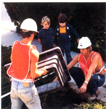
Construction begins in Garden Grove, California. Two young, interested supervisors look on.
