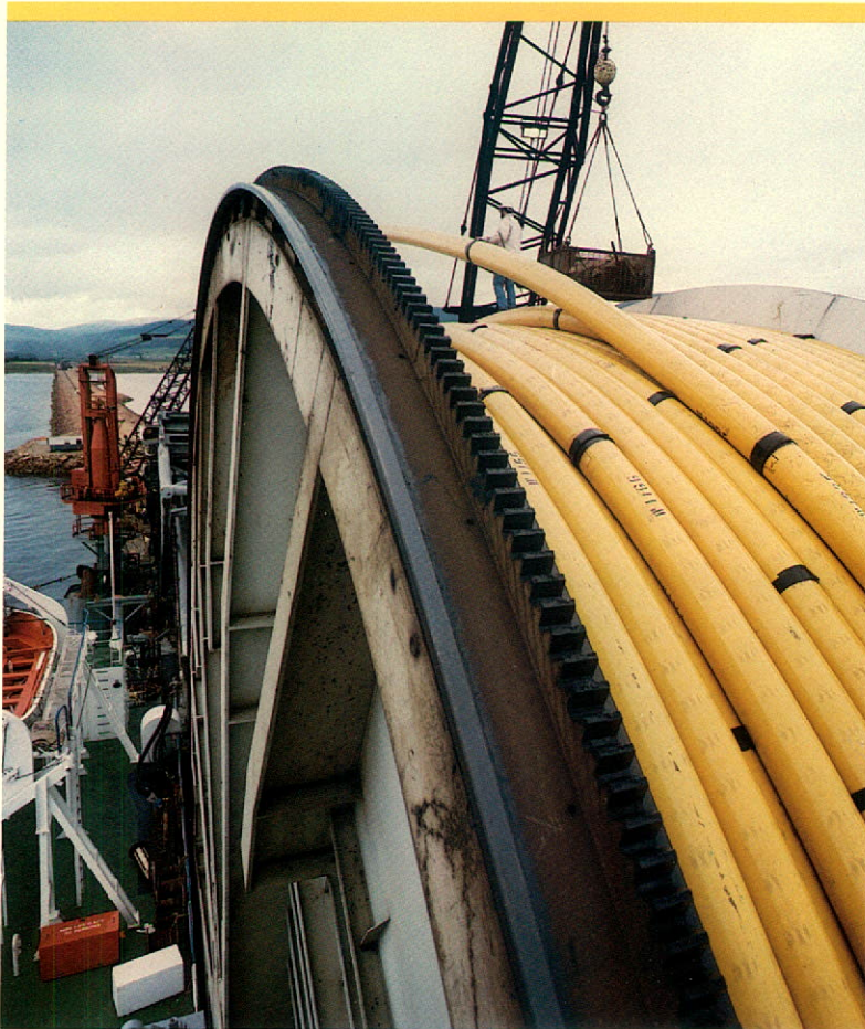
During the 1985 Balmoral field installation program, this giant spool aboard the reel ship Apache fed out nine miles of 14-inch export pipeline in a 40-inch deep trench specially dug on the seabed. It links the template with the Brae-Forties trunkline to the British mainland
