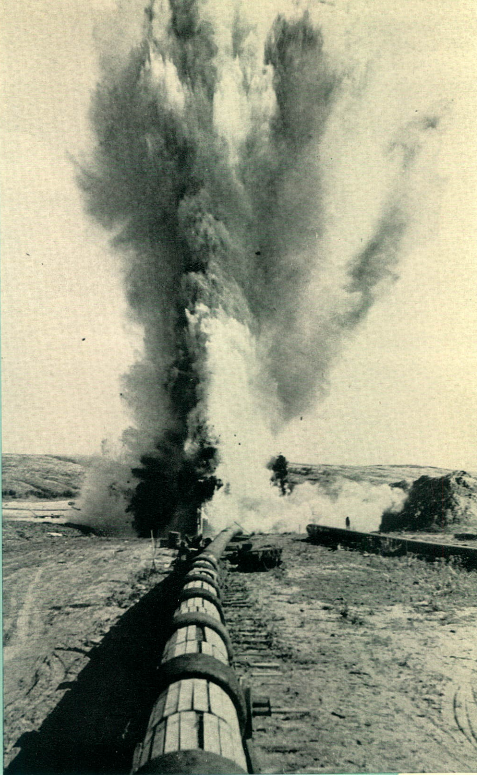
Blasting on the right-of-way for the second crossing of the South Saskatchewan River.
