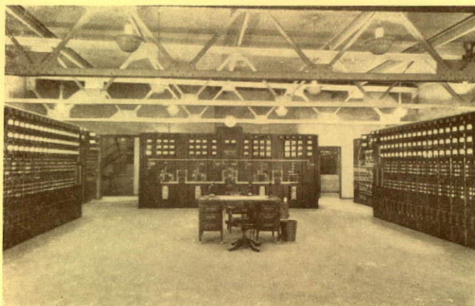
Operating room of Vallée Street Electric Distribution Station showing switchboards and con- trol devices — Montreal
