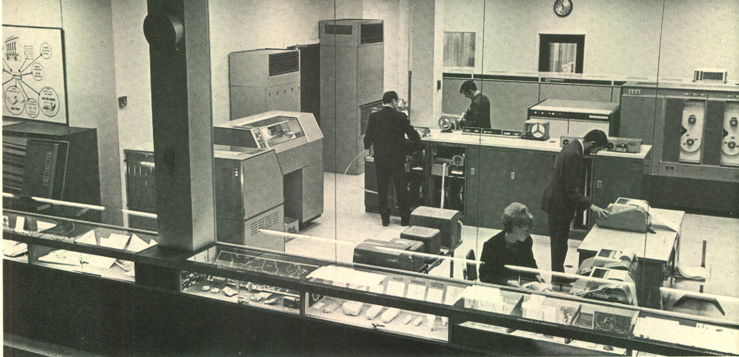
The computer room's serene appearance belies its vital importance to the functioning of an efficient marketplace.
