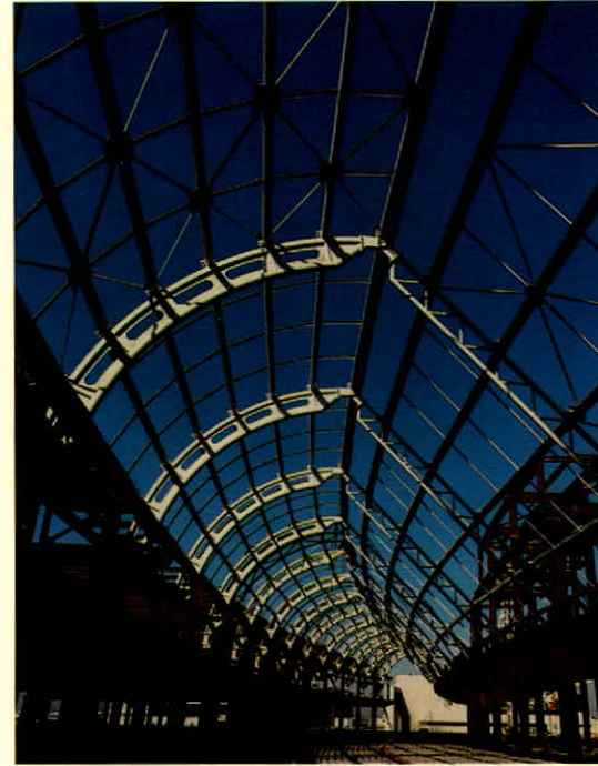
Steelwork fabricated and erected by Canron at Terminal 3 of Lester B. Pearson International Airport.
