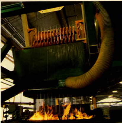
Zinc coated steel wire moves at high speed to the cooling tower.
