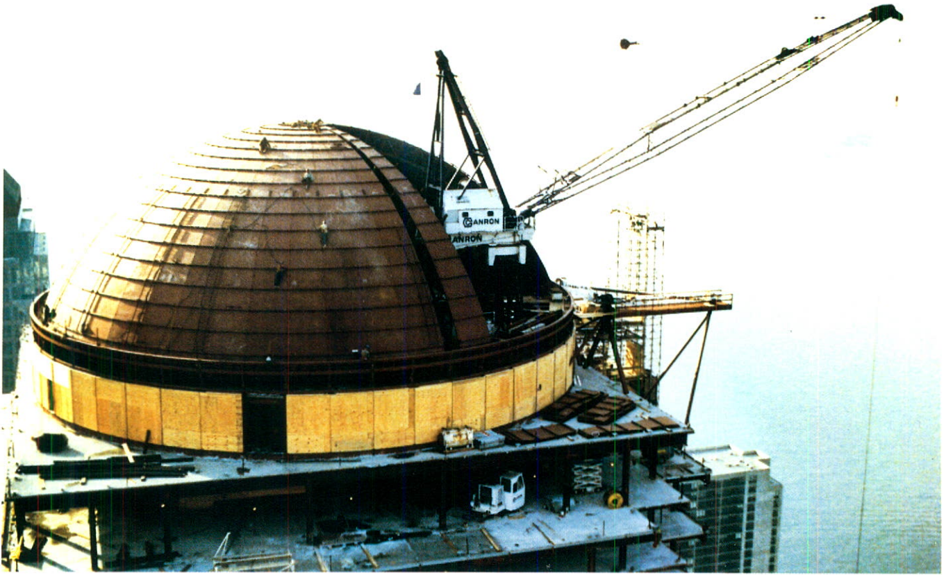
Canron's structural steel division had a major role in the construction of New York's Battery Park.
