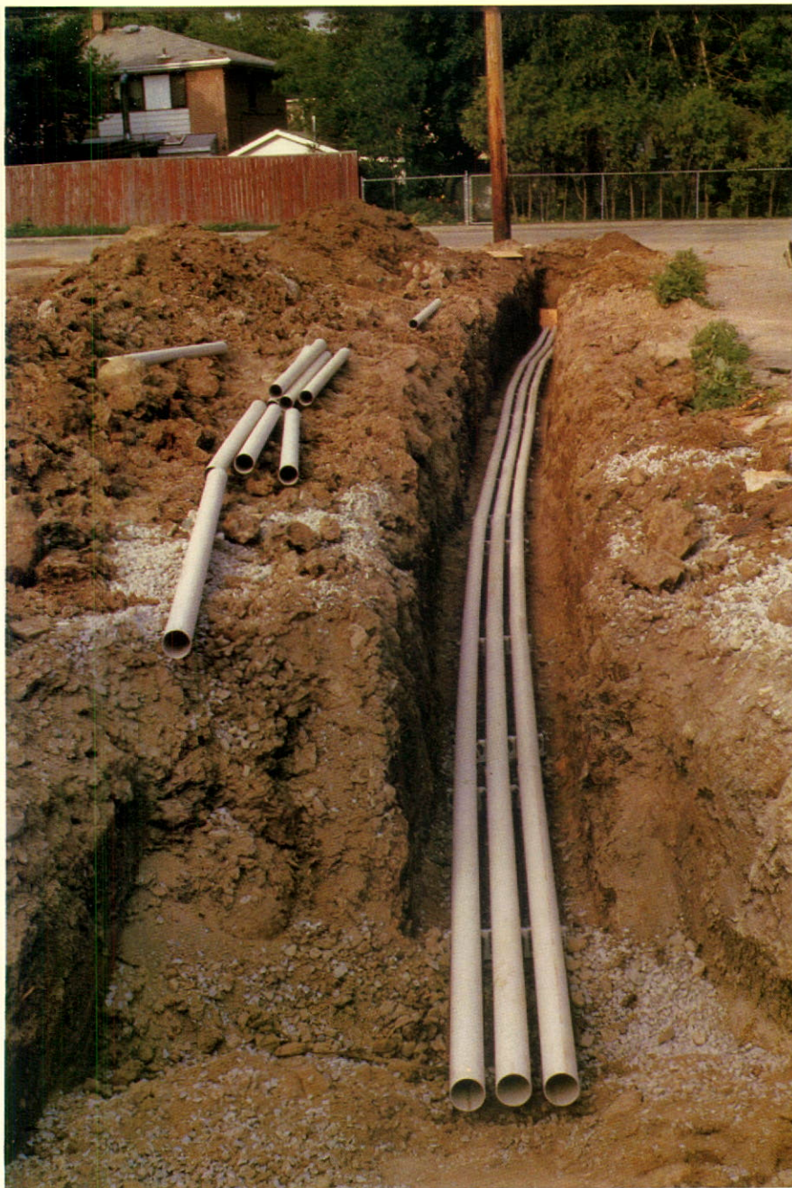
Plastic pipe is Canron's fastest growing product line. This installation is in a Canadian housing subdivision.
