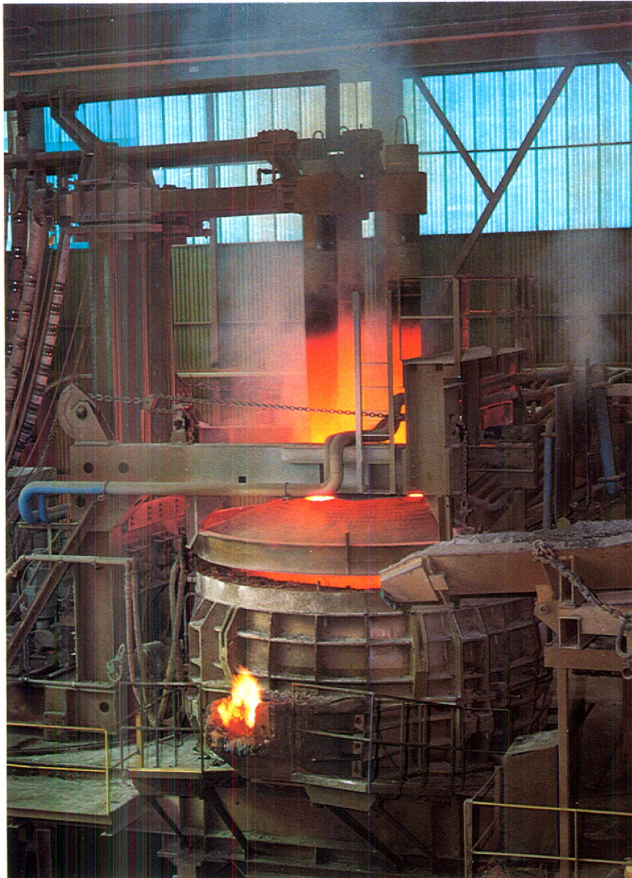
▲ Electrodes being raised prior to charging one of the electric furnaces at L'Original.
