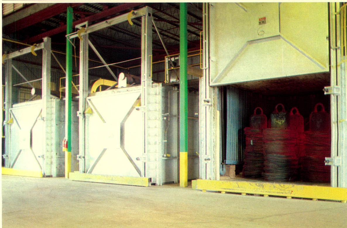
Part of a large bank of annealing furnaces where finished wire is heated and cooled under ▲ controlled conditions.
