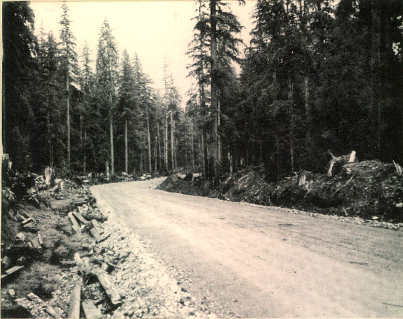
Mainline road at Juskatla, 32 feet wide. Over 9 miles of main road and 6 miles of branch roads have been opened up to date. Roadbed constructed to carry 100 ton loads.
