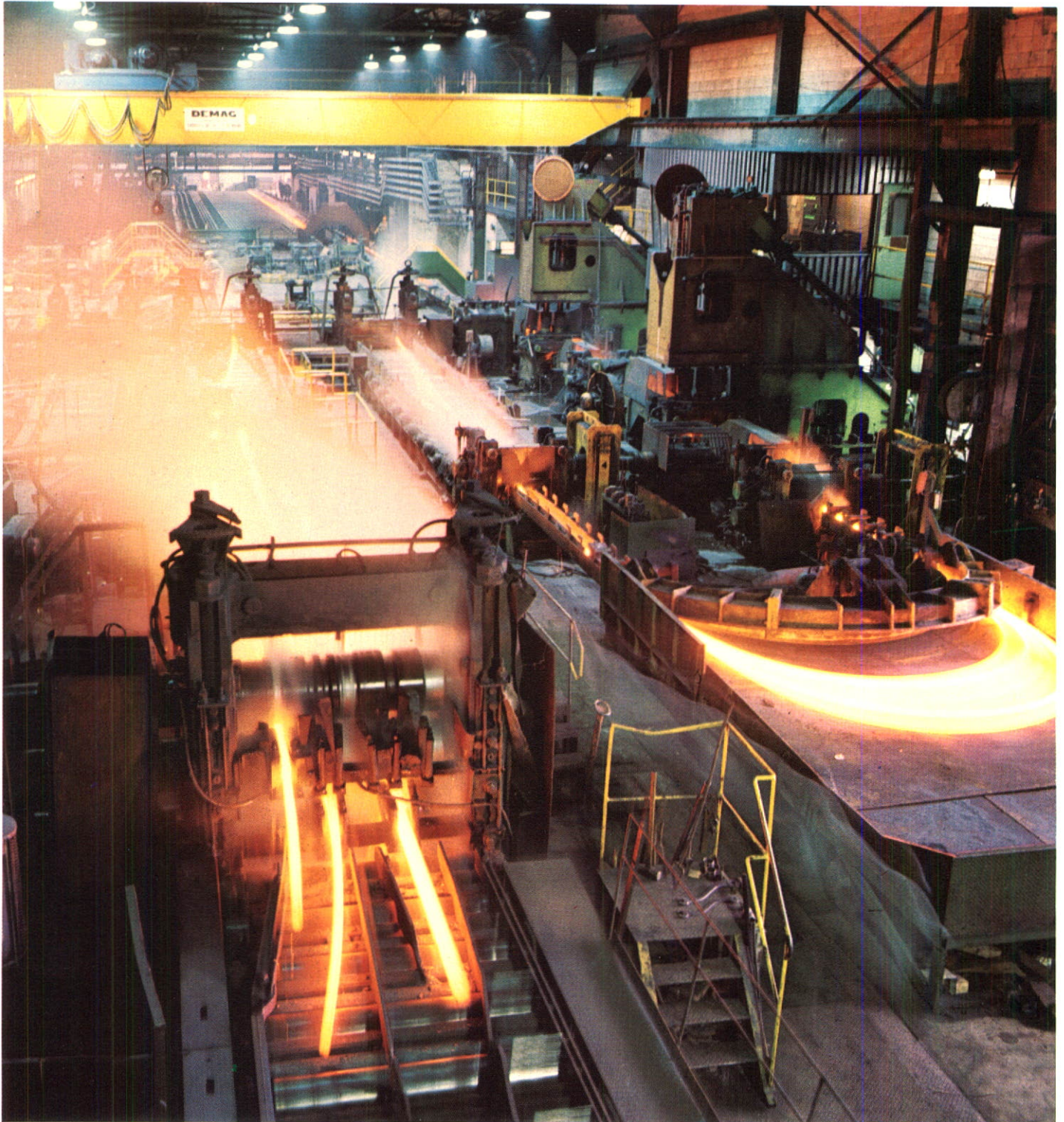
Steel passing through the 21" roughing mill breakdown stand, the first stand of the mill. Steel bars can be seen progressing through the mill to reach the cooling bed at the far end of the mill.
