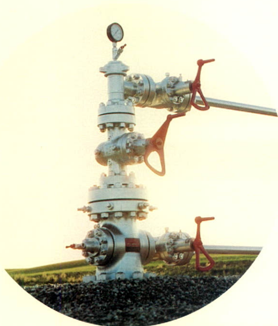
Producing Gas Well — Cessford, Alberta.
