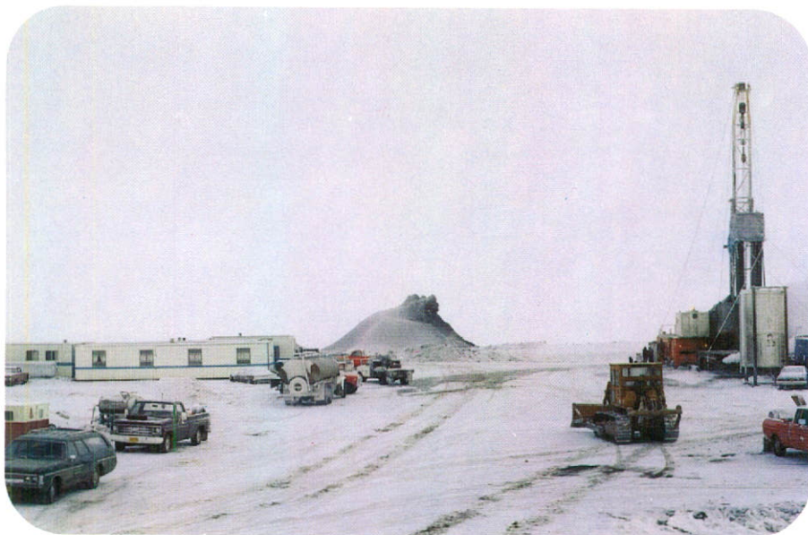
Cessford Project - Relief well in foreground, large mound formed by blowout well in background.
