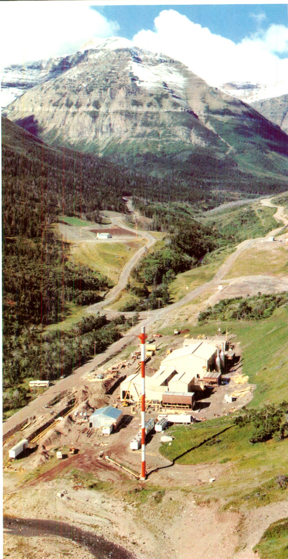
A compressor station under construction in the Waterton natural gas field in Alberta. This station pumps gas to the Waterton plant and came on stream in 1978.
