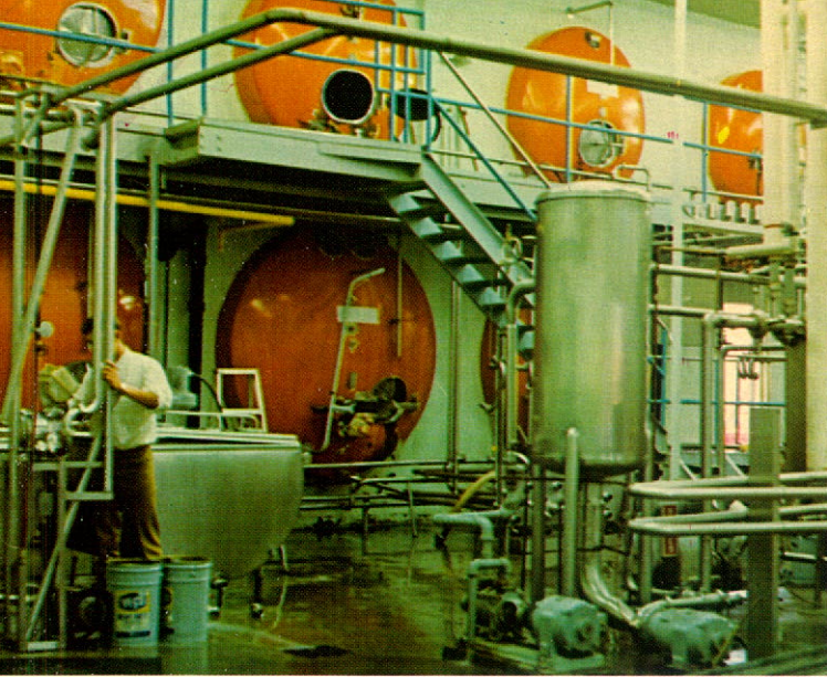
Above: NOCA DAIRY, VERNON. Bulk milk tanks in centralized dairy plant.
