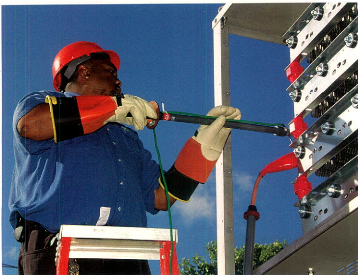
Caribbean Utilities is one of the most reliable and efficient utilities in the Caribbean region.
