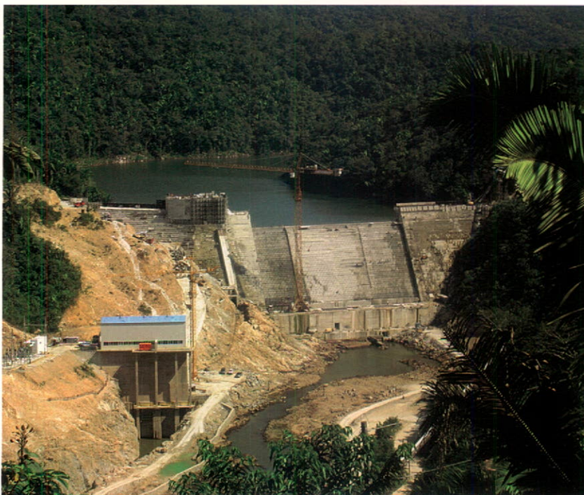
The US$53 million 19-MW Vaca hydroelectric generating facility on the Macal River in Belize will be commissioned in March 2010.
