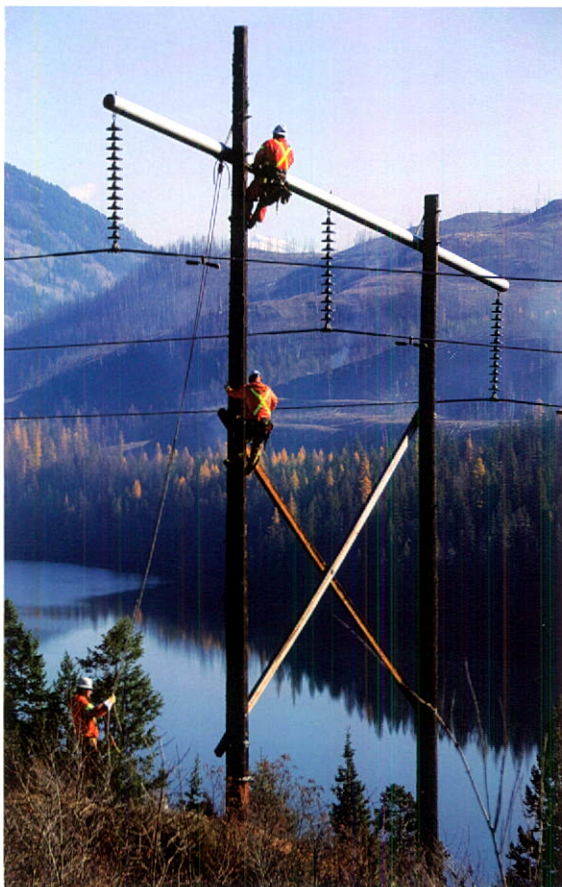
The $110 million Okanagan Transmission Reinforcement Project is the largest capital project ever undertaken by FortisBC.
