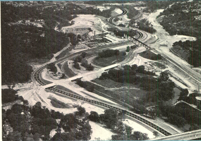
Bayview Avenue Extension, designed by Fenco-Harris as a collector-distributor road for Don Valley Parkway for the Municipality of Metropolitan Toronto, Geo. O. Grant, P.Eng., Commissioner of Roads.
