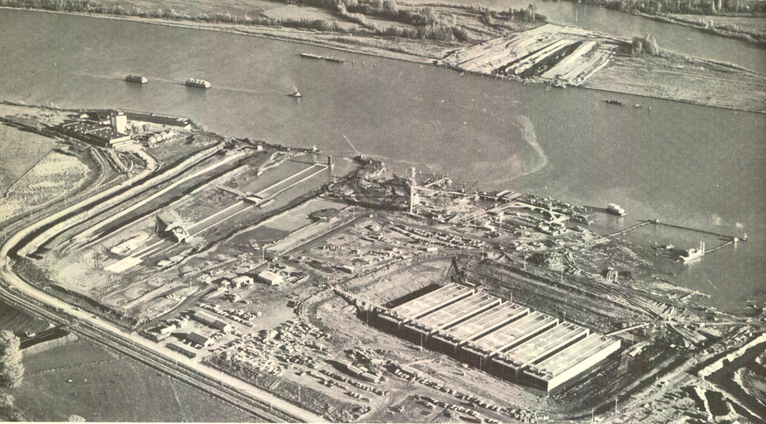
Aerial view showing construction of the Deas Island Tunnel under the Fraser River designed by FENCO in collaboration with Christiani & Nielsen for the British Columbia Toll Highways and Bridges Authority. At each shore are the approach ramps and in the foreground the six 18,500 ton prefabricated tunnel elements which will be floated from their drydock and sunk in position in the river.
