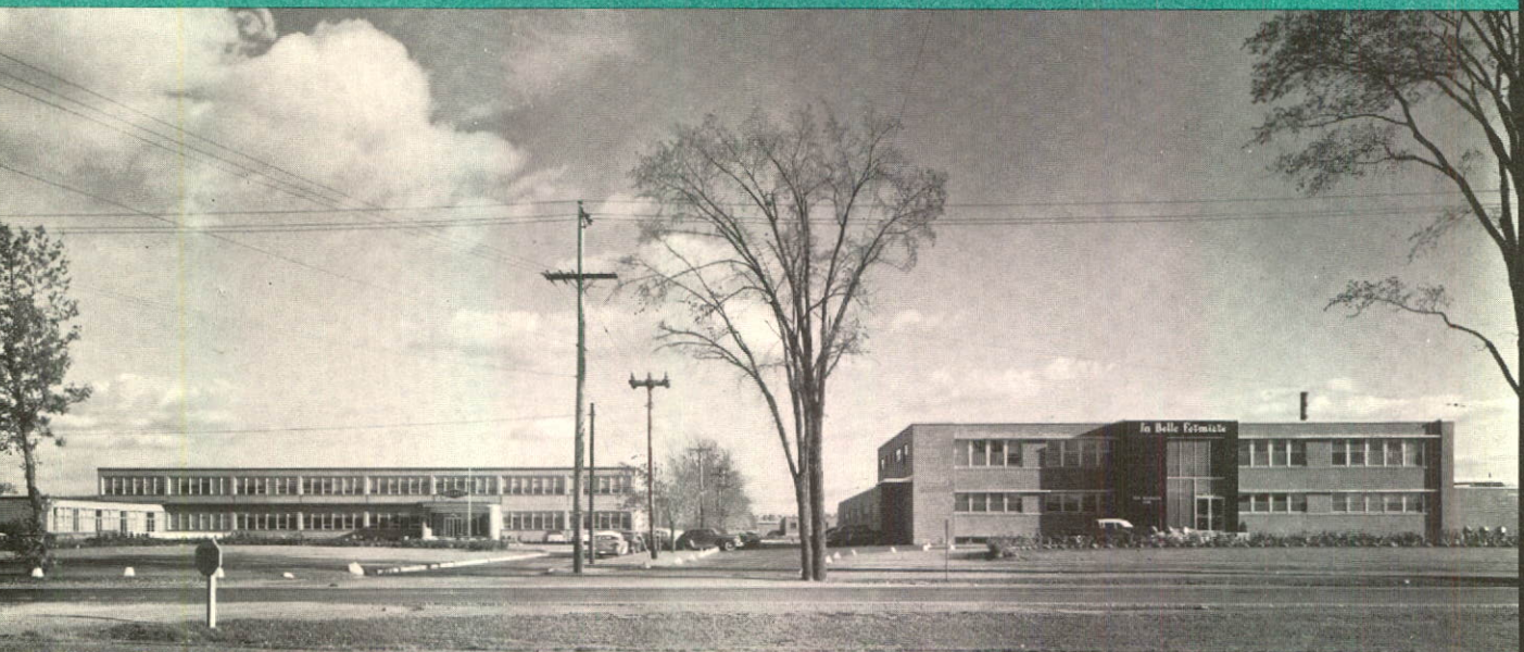
Below: Two plants in Montreal. Gillette Safety Razor Company of Canada Limited. Architects: Ross, Patterson, Townsend & Fish. Noe Bourassa Limitée. Architects: A. Campbell Wood and Hugh W. Blachford.
