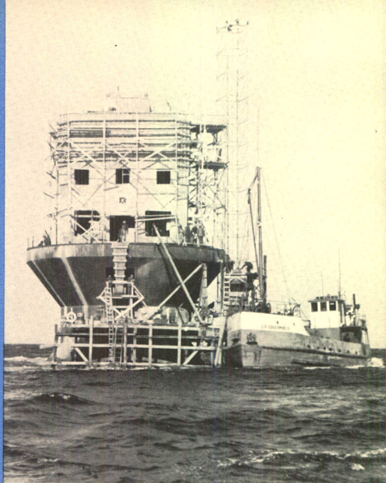
White Island Reef Lighthouse in the St. Lawrence River for Department of Transport, Canada.
