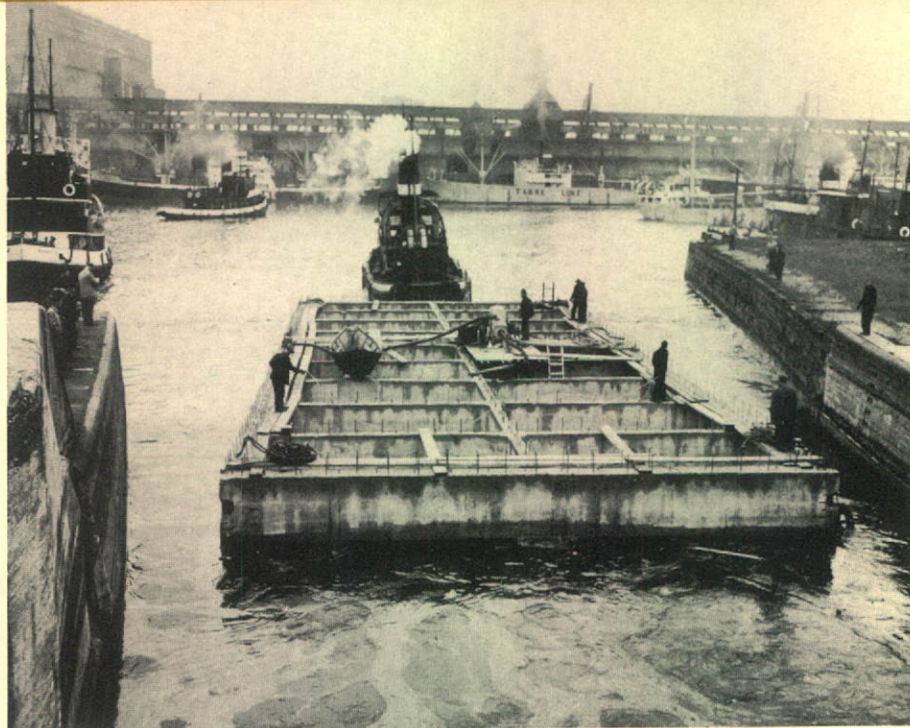
1,100-ton reinforced concrete crib being towed to wharf site in Montreal Harbour for National Harbours Board.
