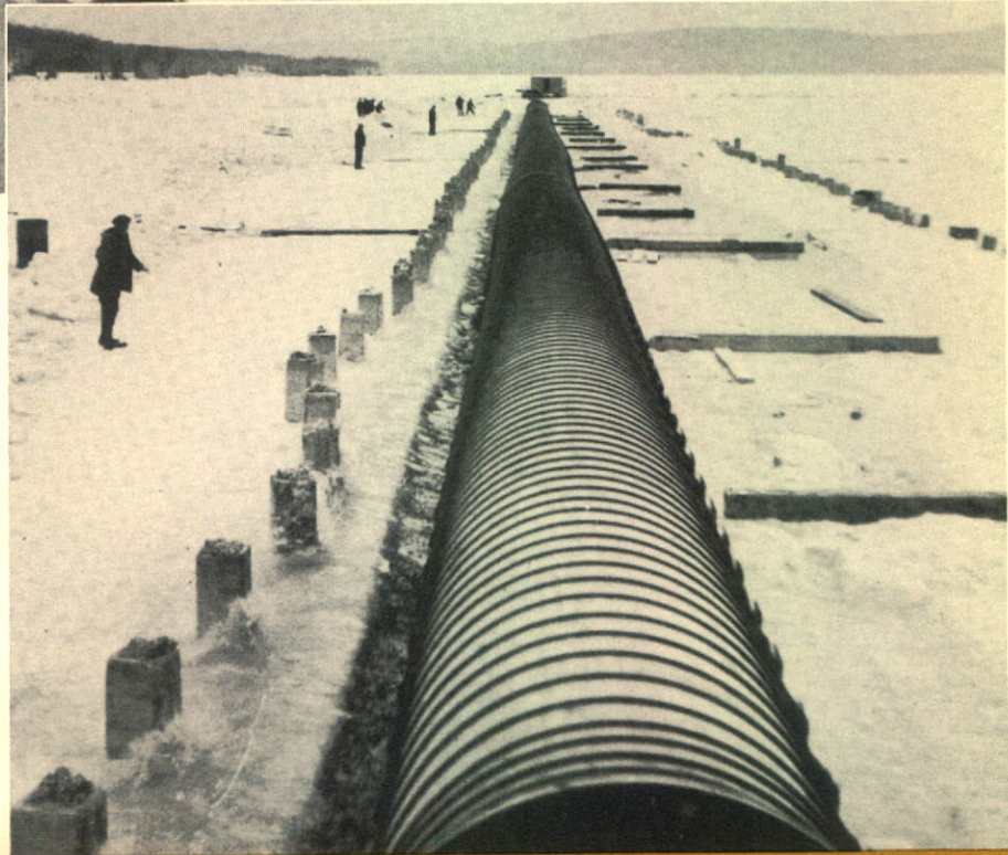
460-foot section of wood stave pipe rigged on ice is rolled into channel on Lake Wayagamack. 3,725 lineal feet of 66-in. diameter pipe for water intake for Town of La Tuque, Quebec. Design by Foundation.
