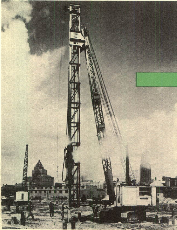
Driving piles for warehouse, Liquor Control Board of Ontario. Equipment was specially designed by Foundation's engineers. Architects, Mathers and Haldenby
