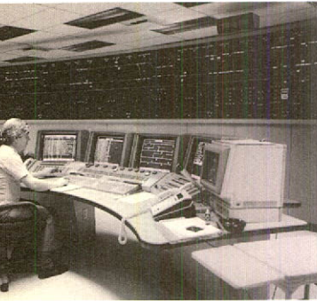
The future Los Angeles subway signed an agreement for the S.T.C.U.M.'s «Ener-Aux» software program, which it will use to distribute electric power and control auxiliary equipment.
