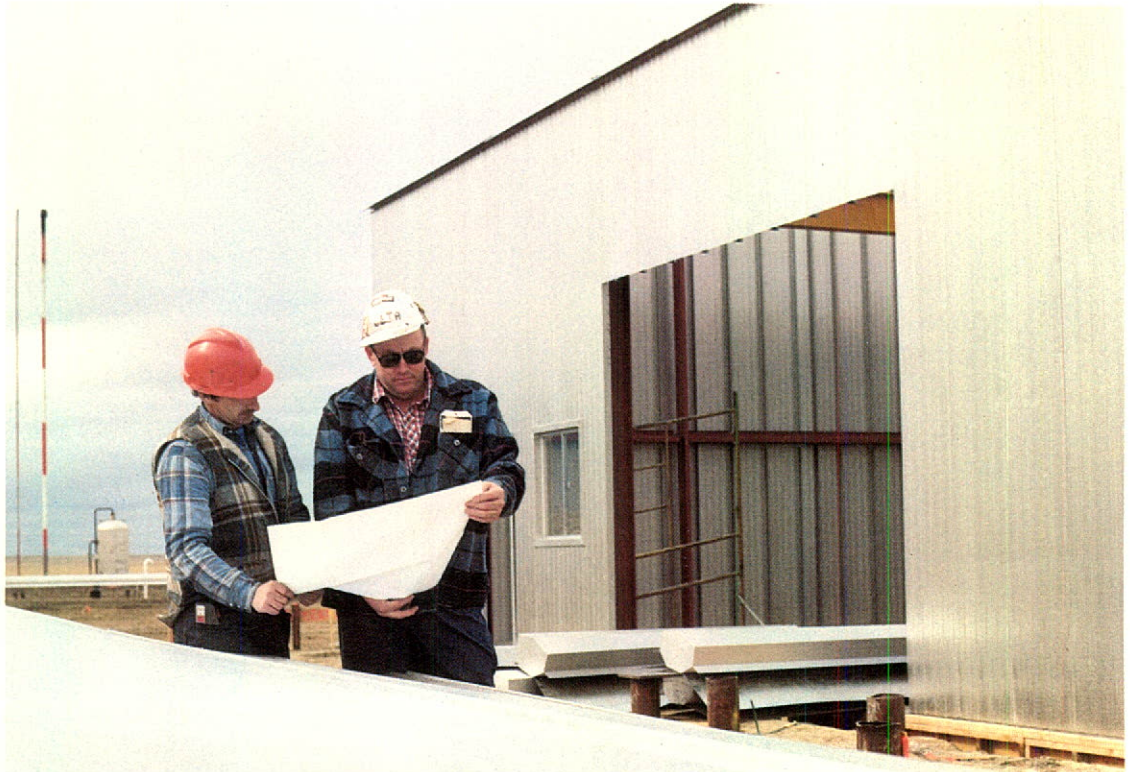
Carbon dioxide extraction facilities under construction at the Turin natural gas plant, Retlaw area. The carbon dioxide will be injected into the Upper Mannville "V" Pool, three miles to the east, in order to improve production performance and oil recovery.
