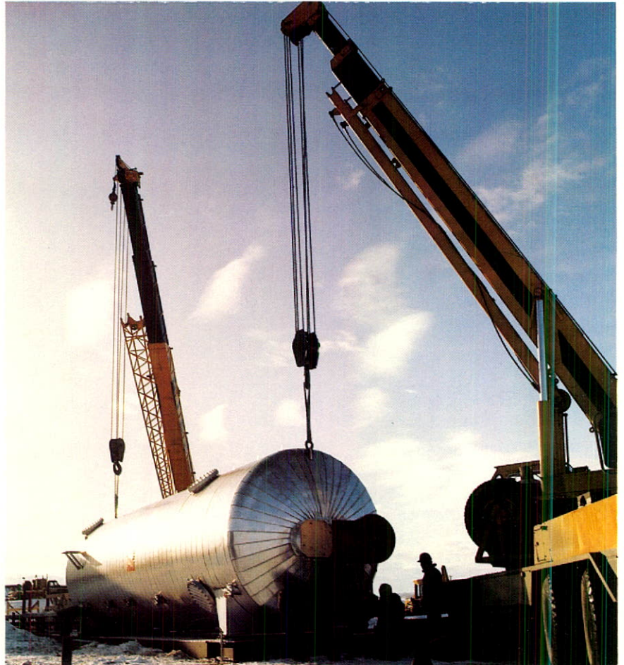
A massive vessel being lifted into place as part of the new cleaning plant which came on stream late in the first quarter of 1984.
