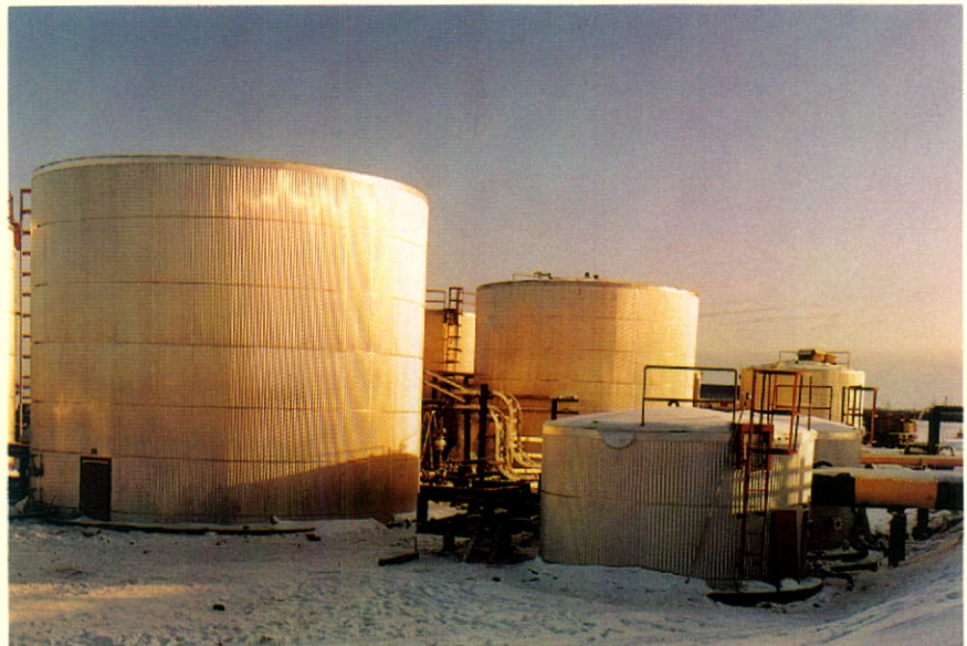
Newly constructed storage tanks at Westmin's new oil cleaning plant near Elk Point.
