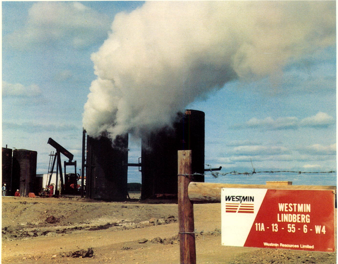
Portable steaming plant at work on tertiary recovery well in the general Lindbergh area.
