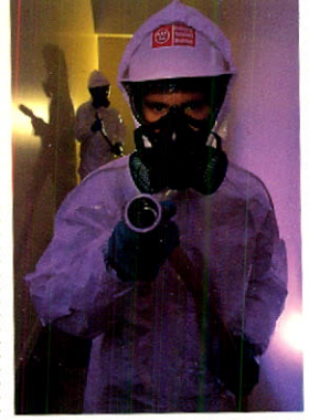
The Environmental Projects Group operates a comprehensive PCB management service to help utility and industrial customers handle PCB equipment and conform to government regulations.
