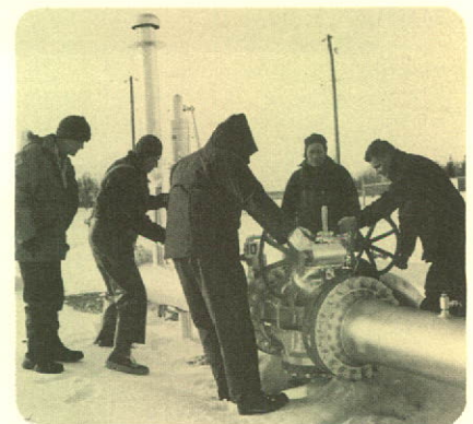
Gas crew services valve at Huntingdon regulating station during winter cold spell.
