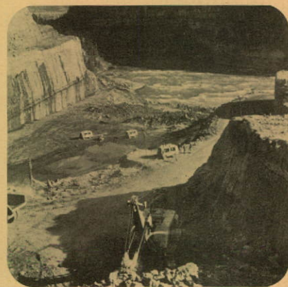
Cofferdam across Peace River will direct waters through this 800-foot channel to tunnels, bypassing the site of the Portage Mountain Dam.
