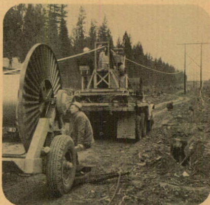
Stringing conductor on the first stage of the Bridge River-Prince George transmission line.
