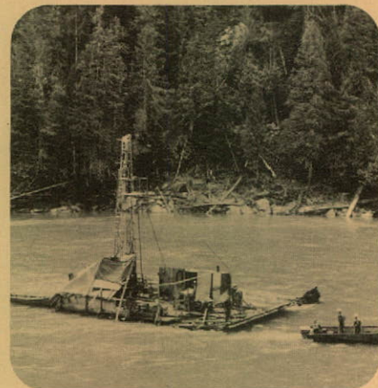
Barge-mounted drilling rig investigates foundations for the proposed Mica Creek dam on the Columbia River about 90 miles north of Revelstoke. Operation was part of field surveys and investigations carried out during the past year.
