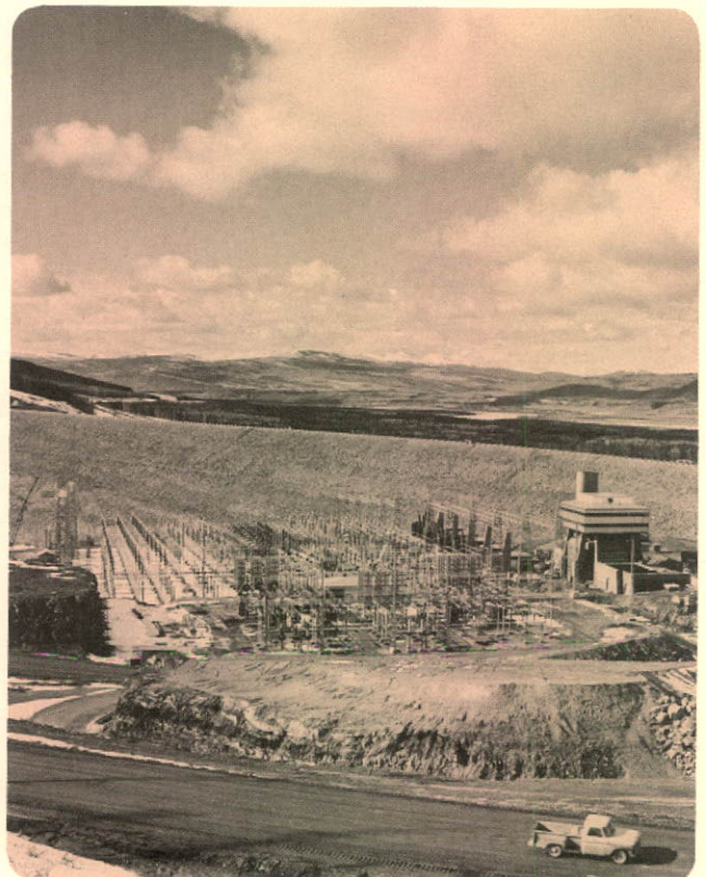
High-voltage, long-distance transmission will begin at switchyard.
