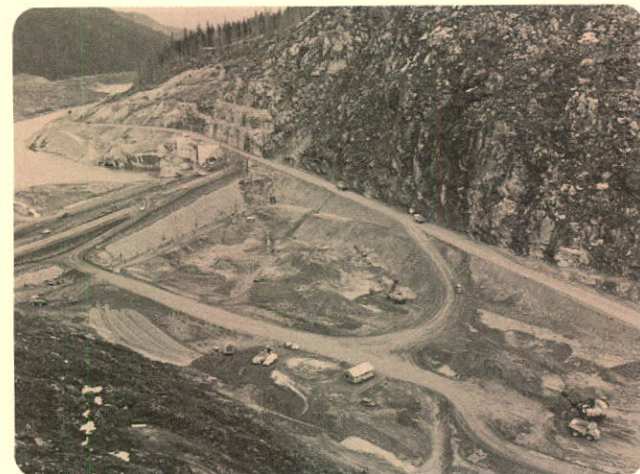
Excavation of river bed will provide solid rock base for Mica Dam.
