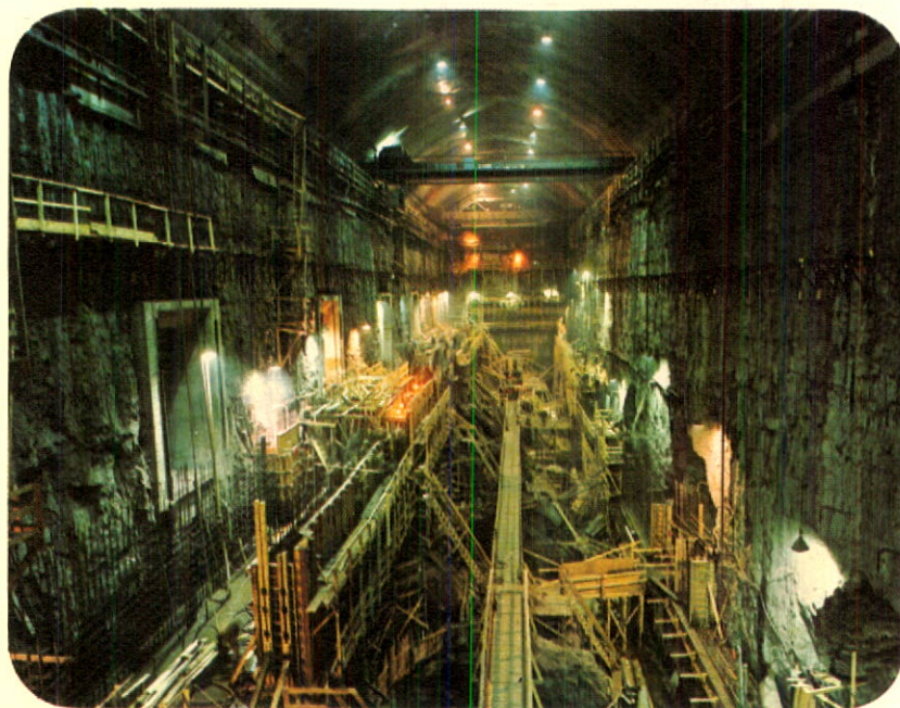
The world's largest underground hydro-electric power plant takes shape at Portage Mountain, Peace River Project. The powerhouse cavern measures 890 feet in length, 67 feet in width and up to 150 feet in height.
