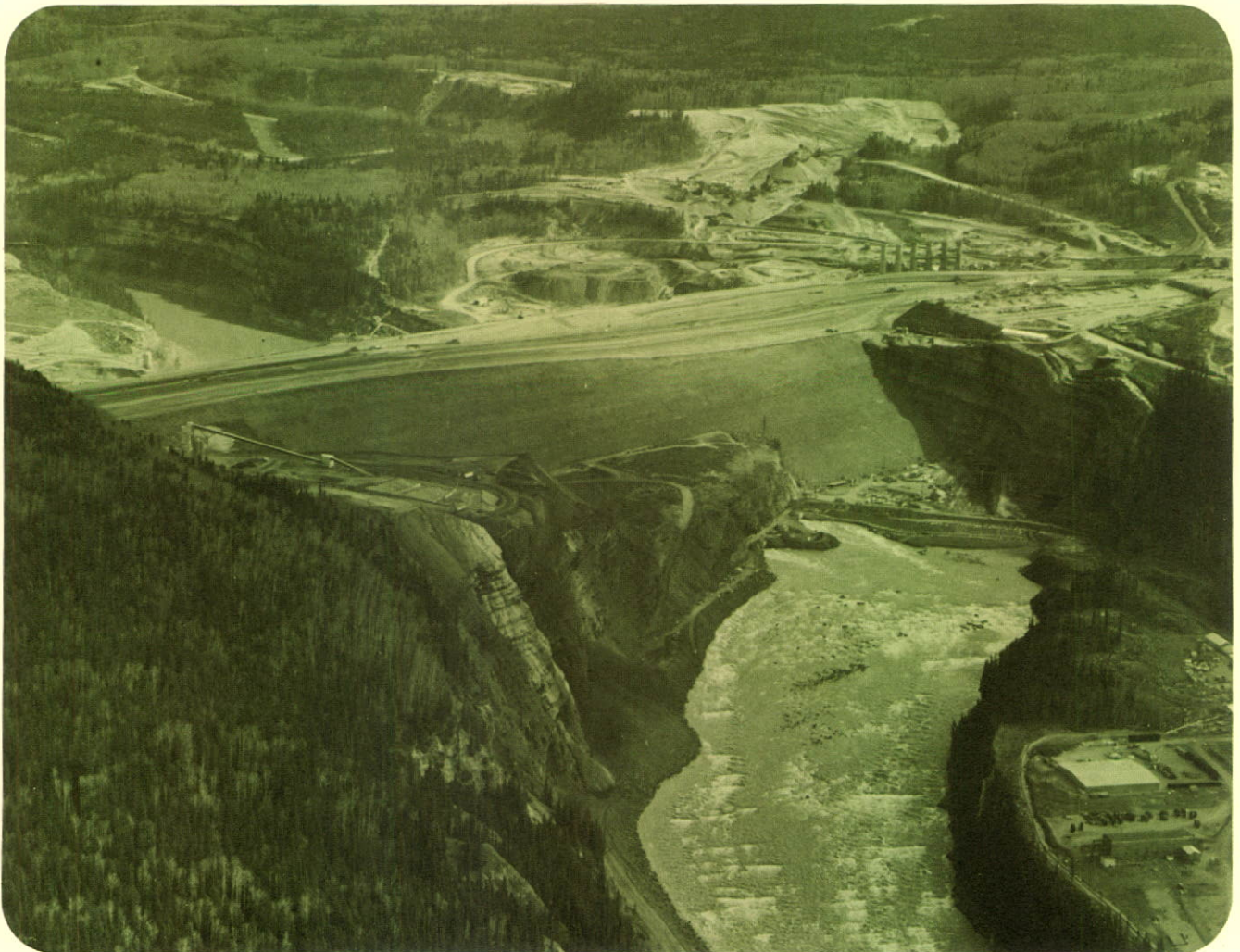
450 feet high at the end of 1966 construction season, Portage Mountain Dam will reach height of 600 feet above river bed when completed.
