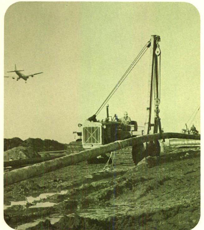
This 8-inch pipeline is part of distribution system that will supply natural gas to the new terminal at Vancouver International Airport.
