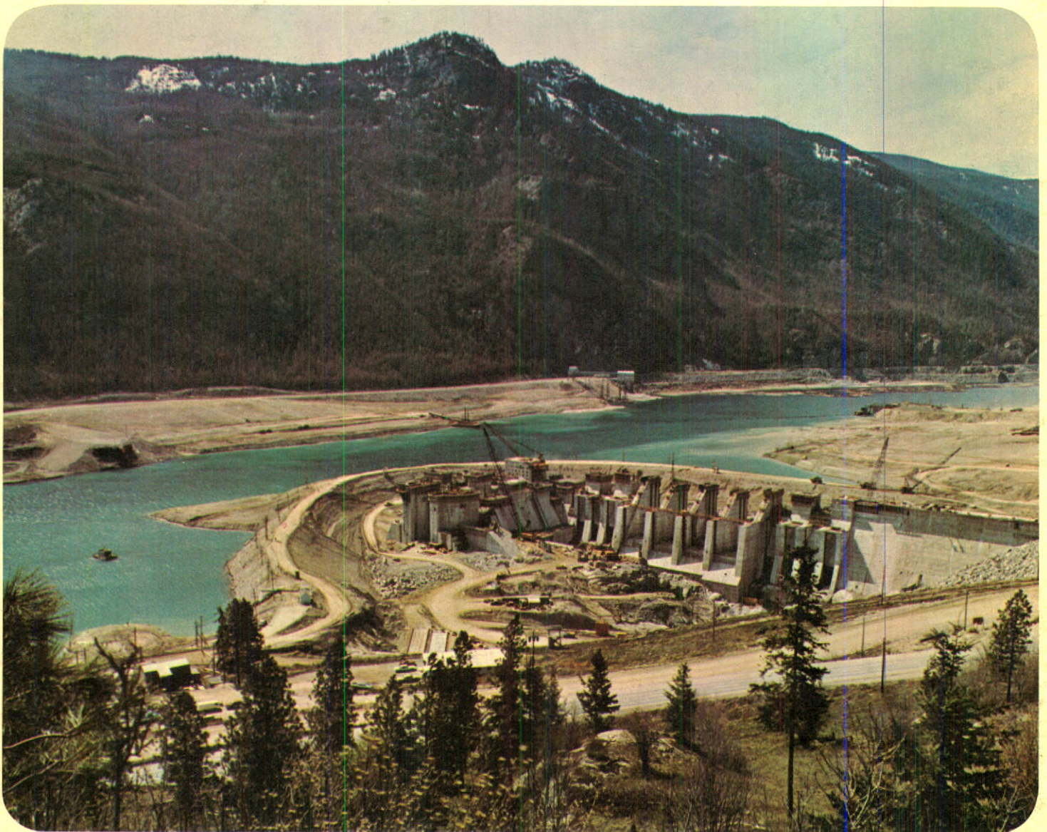
Arrow Dam navigation lock and reservoir discharge structures being constructed within a horseshoe-shaped cofferdam extending into the Columbia River.
