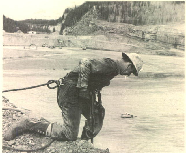
Driller at work on left bank escarpment, high above Portage Mountain dam site.
