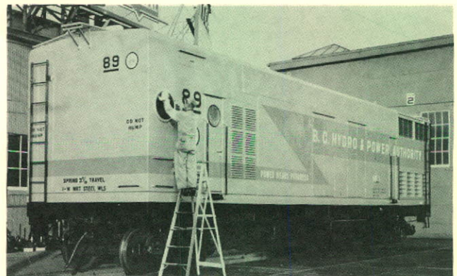
One of the Authority's seven 1,000 kw power generating rail cars; each can be moved quickly to any point on the Province's railway network.
