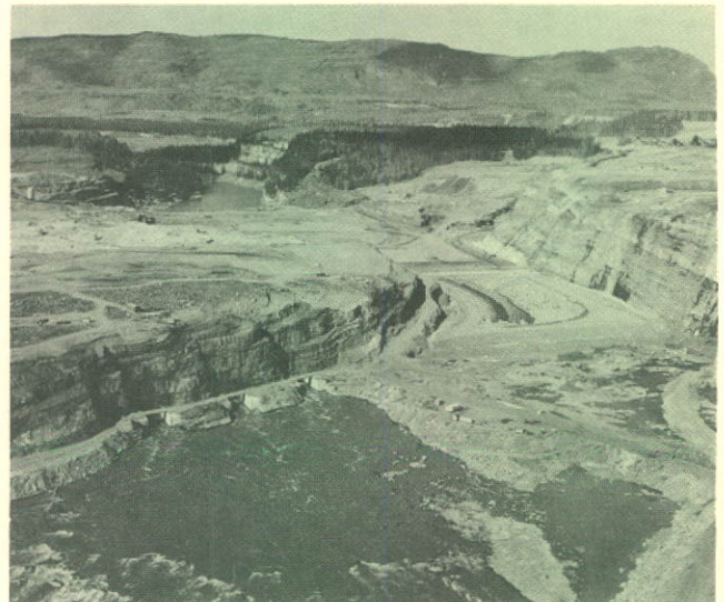
Aerial view of the Peace River Project, with outlets of diversion tunnels in left foreground.
