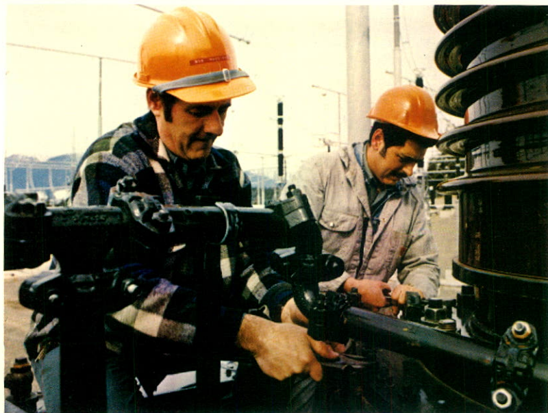
Subforeman serviceman Bob Maddison (left) and serviceman Don Gallanders working in substation at Terrace.
