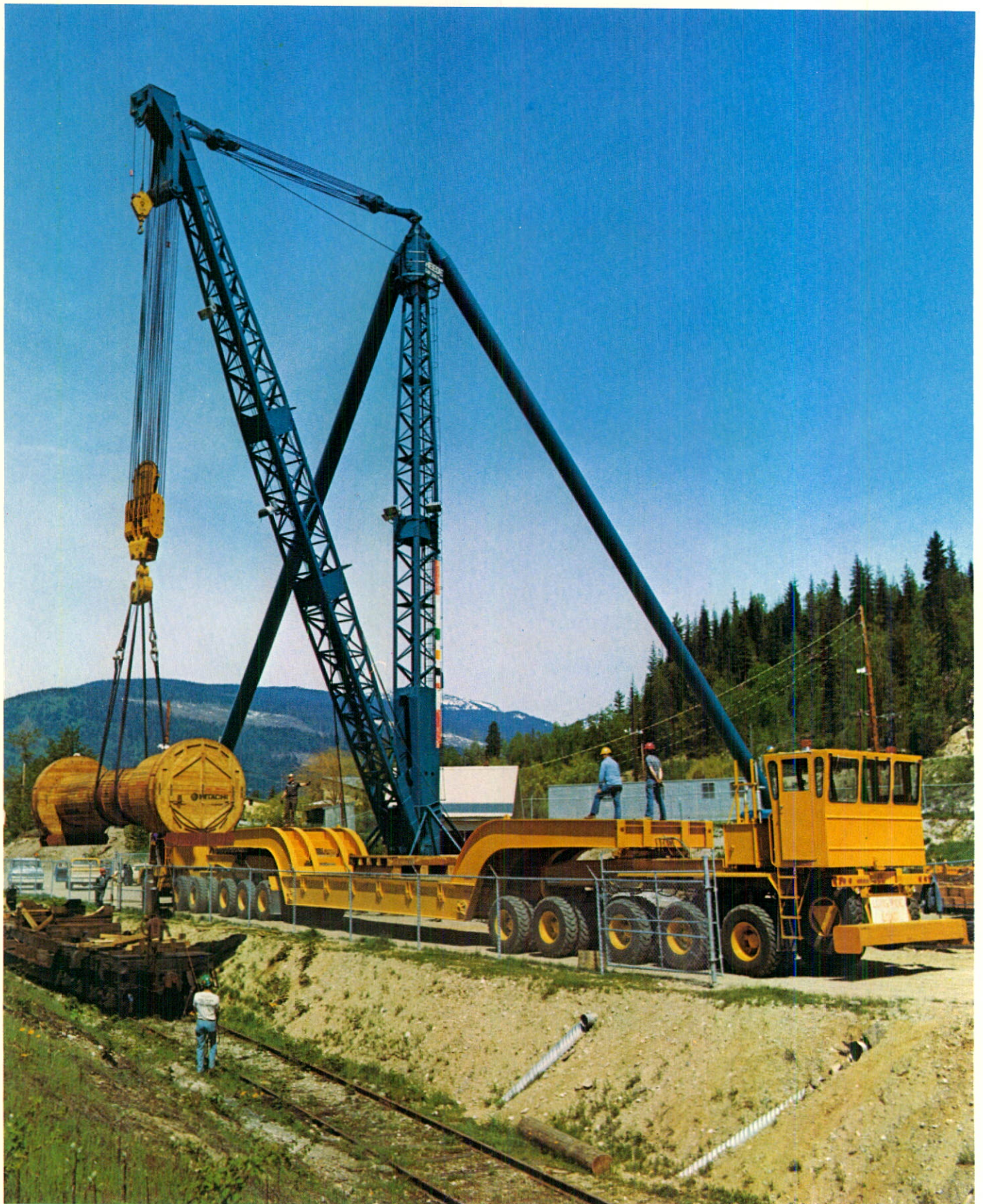
Turbine shaft was transferred from rail car to low-bed trailer at Revelstoke for final leg of trip to Mica.
