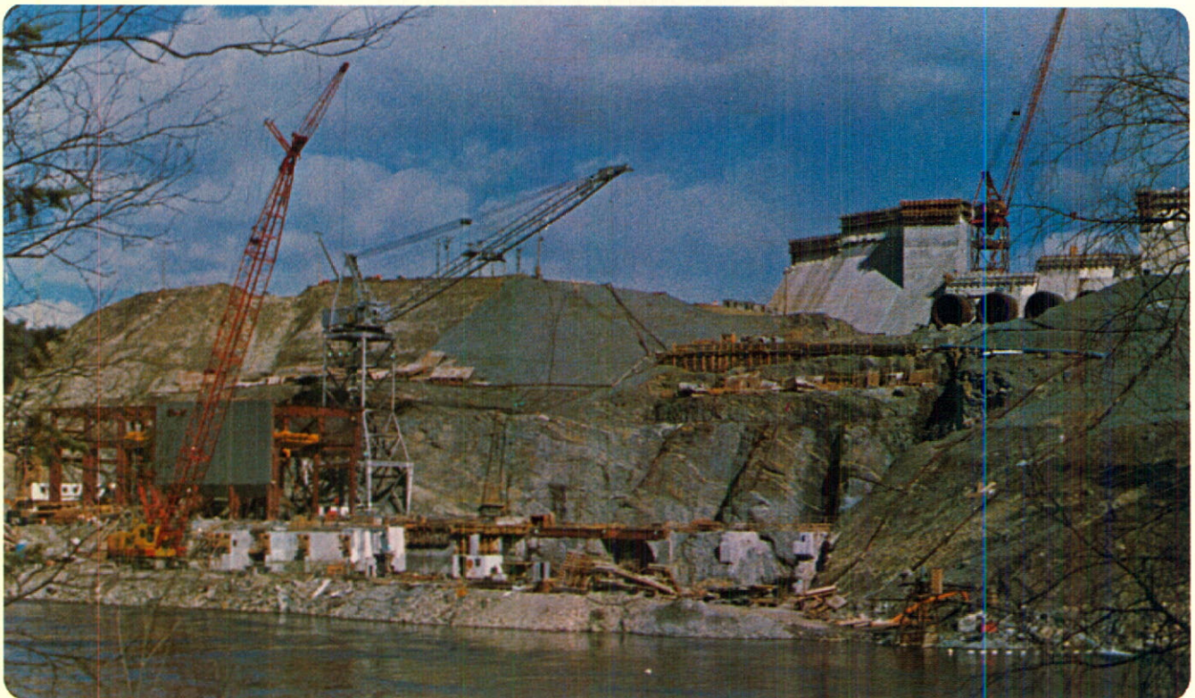
Construction of three-mile-long Kootenay Canal was substantially completed and work proceeded satisfactorily on other aspects of the development. First two generating units are scheduled for service in 1975 and the other two in 1976.
