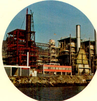
1965 — Third unit at Burrard Thermal.
