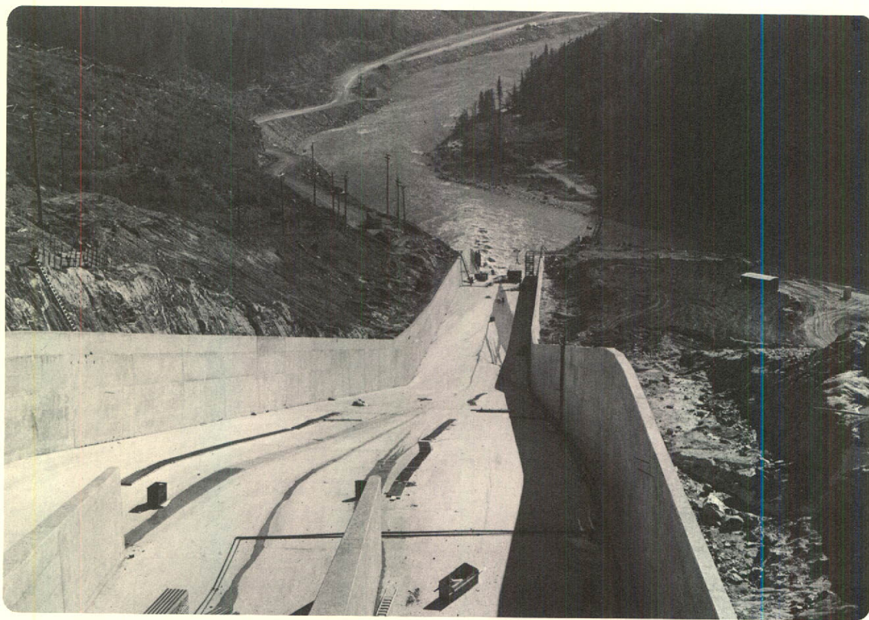
Spillway structure was virtually completed as workmen prepared for final year of construction on huge Mica Dam.
