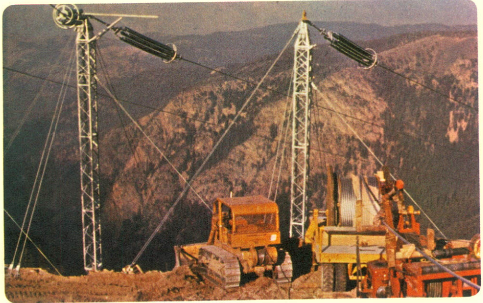
Rough terrain and weather at Mission Ridge posed stiff test for powerline builders.
