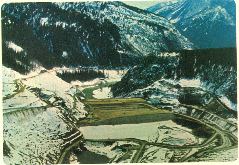
Mica Dam reached a height of 440 feet before annual snows ended construction season.
