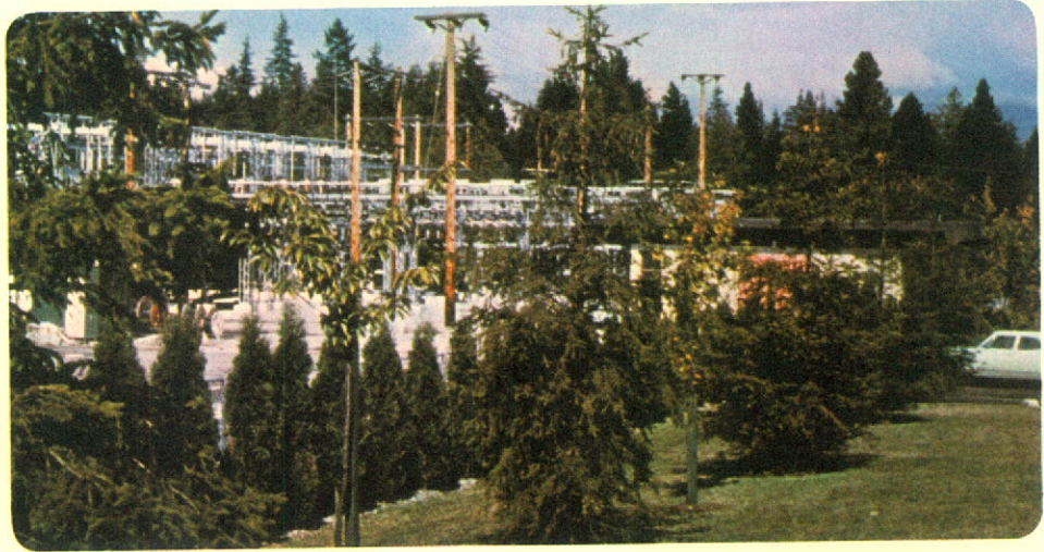
New low-profile design of B.C. Hydro substations is functional and pleasing to the eye.
