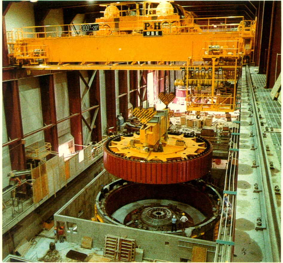
First two generating units at Seven Mile hydroelectric project near Trail came on line well ahead of schedule.
