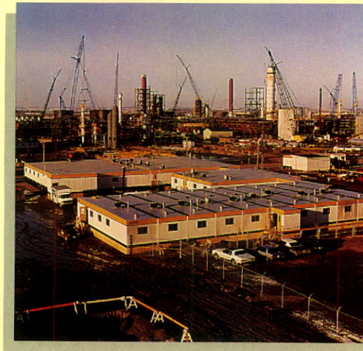
▲ At the Bi-Provincial Upgrader site in Lloydminster, Alberta, ATCO supplied and installed the office complex.
