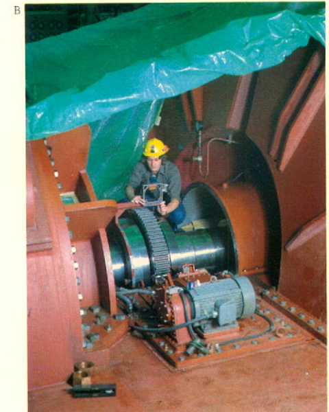
A. Alberta Power's Battle River Generating Station near Forestburg, Alberta. B. $118 million was spent on the construction of the 375-megawatt addition to the Battle River Generating Station.
