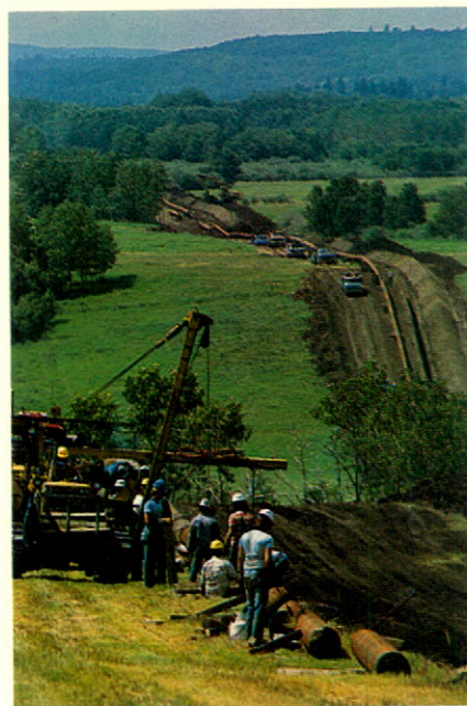
Above: Crews lay transmission pipeline, one of the projects totalling $37 million during the year to meet growing service obligations of Canadian Utilities Limited. Left, below: A natural gas regulating station in Calgary, typical of numerous installations operated to provide utility service.
