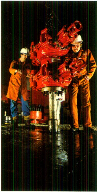
Above: Making certain it's right before it's rented, ATCO Oilfield Equipment shop mechanics inspect a blowout preventer before it is sent to a customer. Throughout western Canada, drilling and well servicing companies rely on equipment from this division. Below, right: An ATCO Well Servicing rig at work in southern Alberta. Similar equipment is located throughout western Canada and the U.S. and one rig now is operating in Australia, enhancing recovery from existing wells and completing new ones.
