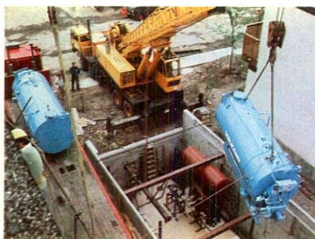
Canada's first low-temperature hot-water heating system is shown being installed for testing in a downtown residential community in Ottawa.
